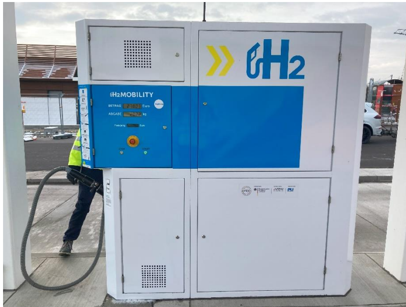
Figure 18. 350 bar HDV refueller at Magdeburg (source: H2M)
